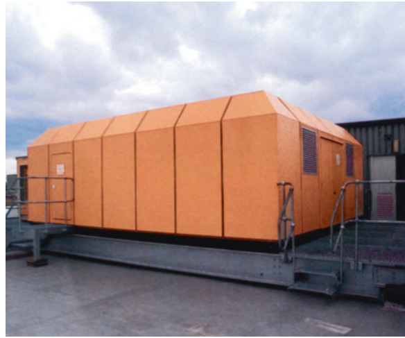
PACKAGED PLANTROOM with SECTIONAL WATER CISTERN and associated equipment
