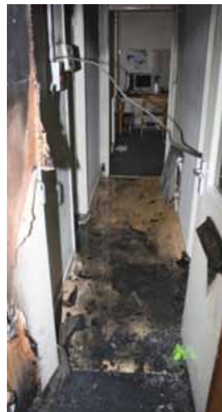
In August 2011 a fire occurred in another Callow Mount block, not the one in which sprinklers were being installed.
