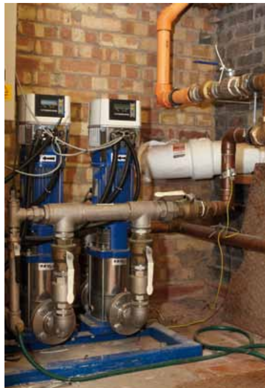
The four internal service mains in the block provided the water for the sprinkler system. Twin electric pumps supplement the service main's supply although, during installation, the mains pressure was tested and the 1.5bar reading at the top floor was in any case judged sufficient for the system.
