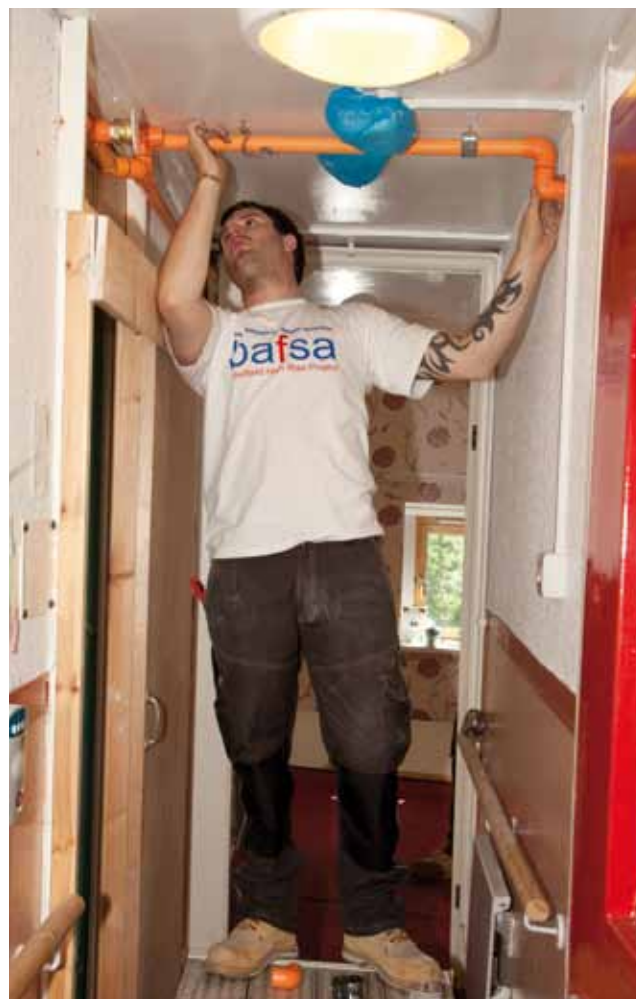
CPVC pipework and related components were the products of choice for the project. Some boxing-in would be necessary for system pipework although, wherever possible, it was hidden within the same concealment as domestic rising mains.
