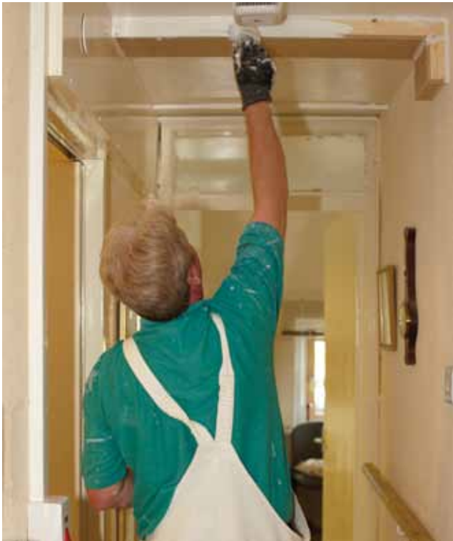
The installation work involved associated carpentry and subsequent redecoration, all carried out with consideration and care in residents' homes.
