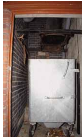
The sprinkler retrofit was planned to protect all the block's flats, lobbies, communal rooms and even the four external bin stores at the bases of the bin chutes (see above). Bin stores are frequently targeted by arsonists.
