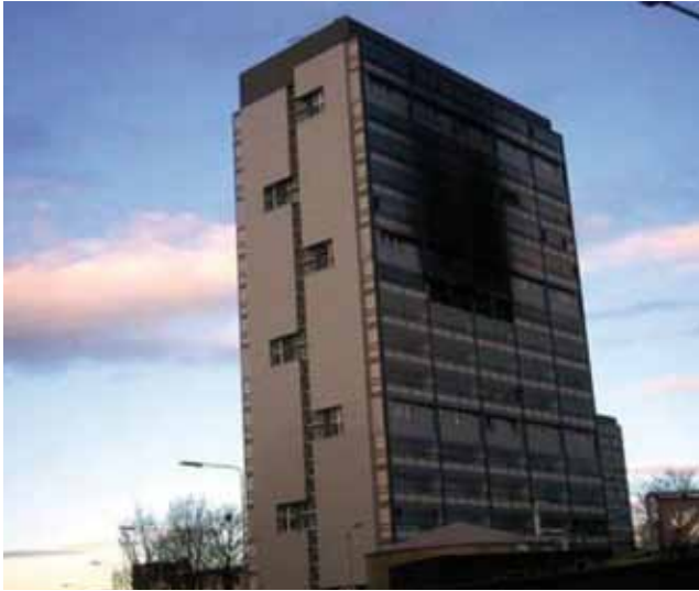
There was a fire at Waddell Court, Glasgow, December 2011 (photo courtesy of Glasgow Housing Association/Strathclyde Fire and Rescue Service).
