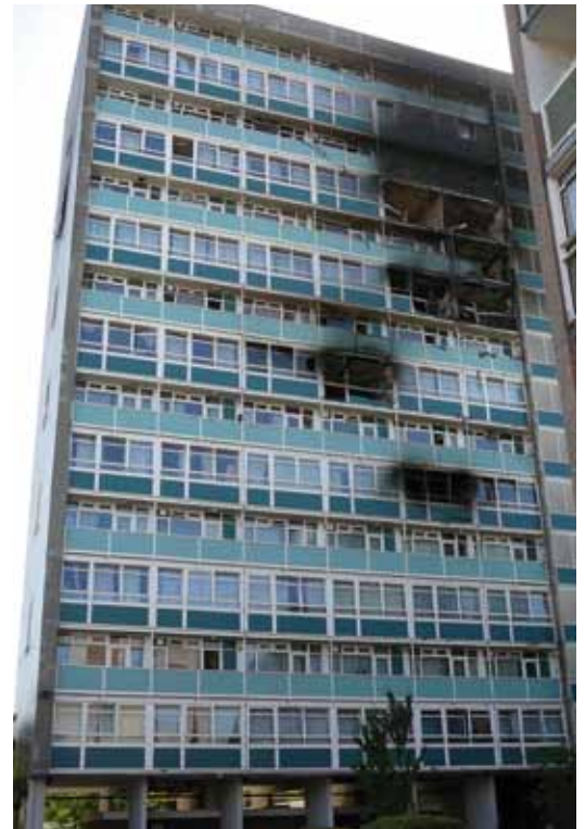
The fire at Lakanal House, Camberwell, London on 3 July 2009 killed 6 people and injured 20 others. The 12-storey tower block was unsprinklered; after the fire all residents were evacuated and rehoused and the block remains empty.
